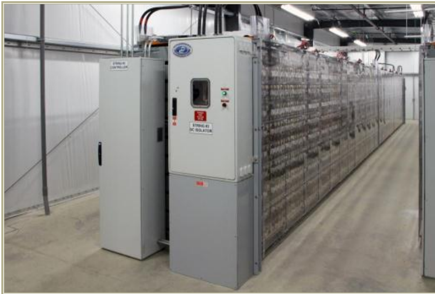
Figure 21: Storage Installation at PJM Regulation Services Project
