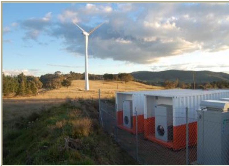
Figure 20: Energy Storage installation at Hampton Park Wind Farm
