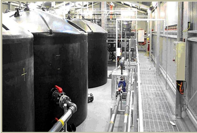
Figure 15: Electrolyte storage tanks comprising the King Island VRB
